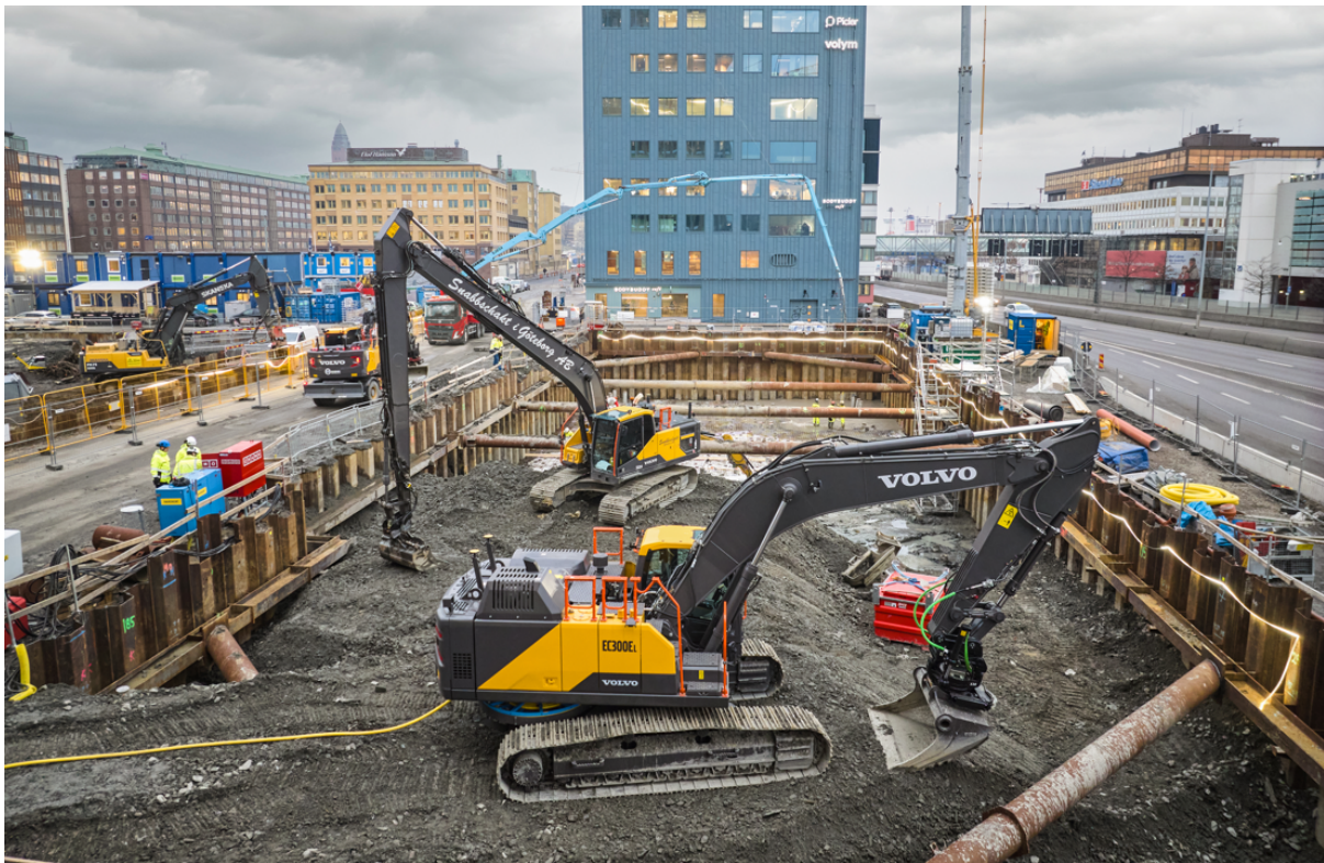
Volvo CE's large 30-ton grid-connected electric excavator formed part of the Electric Worksite tests. Photo: NCC, Joakim Kröger
