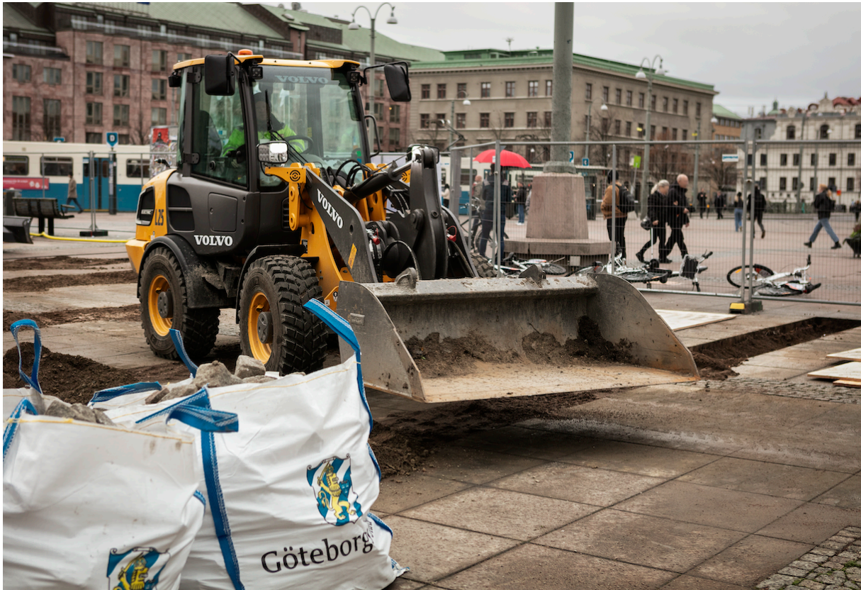
The L25 Electric compact excavator working at Drottningtorget in central Gothenburg. Photo: Electric Worksite.
