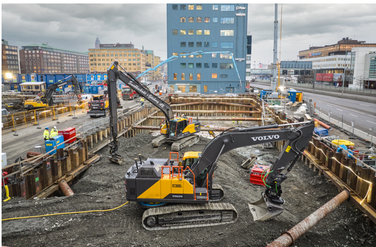
Volvo CE's large 30-ton grid-connected electric excavator formed part of the Electric Worksite tests. Photo: NCC, Joakim Kröger
