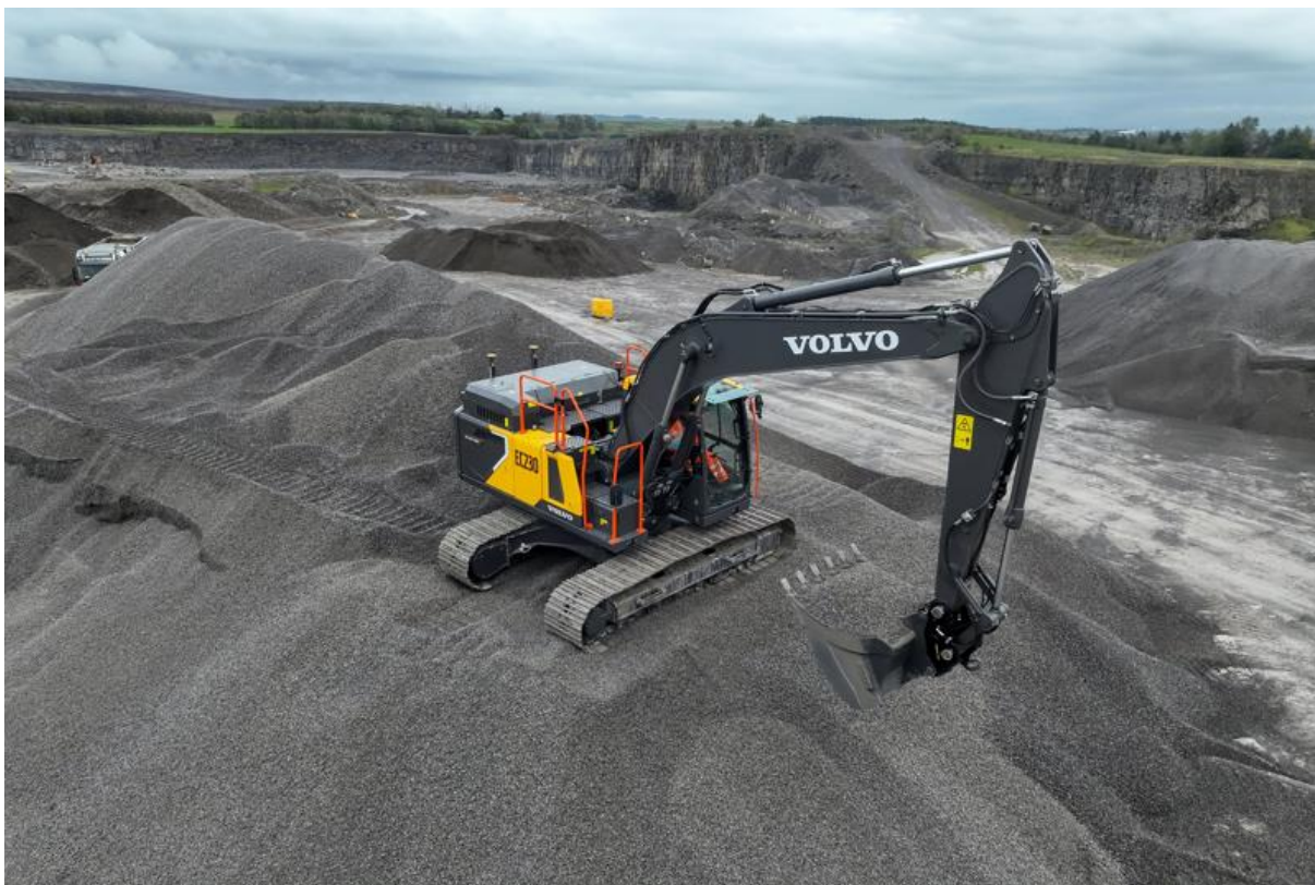
The EC230 Electric excavator has already been put to work on a recent CRH project for Low Carbon Roads
